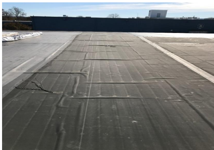
Figure 5. “Mole tunneling” that can result from the thermal expansion and contraction of roofing membrane after installation.
