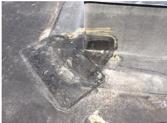
Figure 6 . Uncured pressure-sensitive flashing used to seal the outside corner of a curb to the roof deck. Two pieces of flashing are used with multiple overlapping seams. Sealant has also been used around the edges of the flashing.
